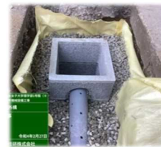
Rainwater infiltration pipe and rainwater infiltration trench
